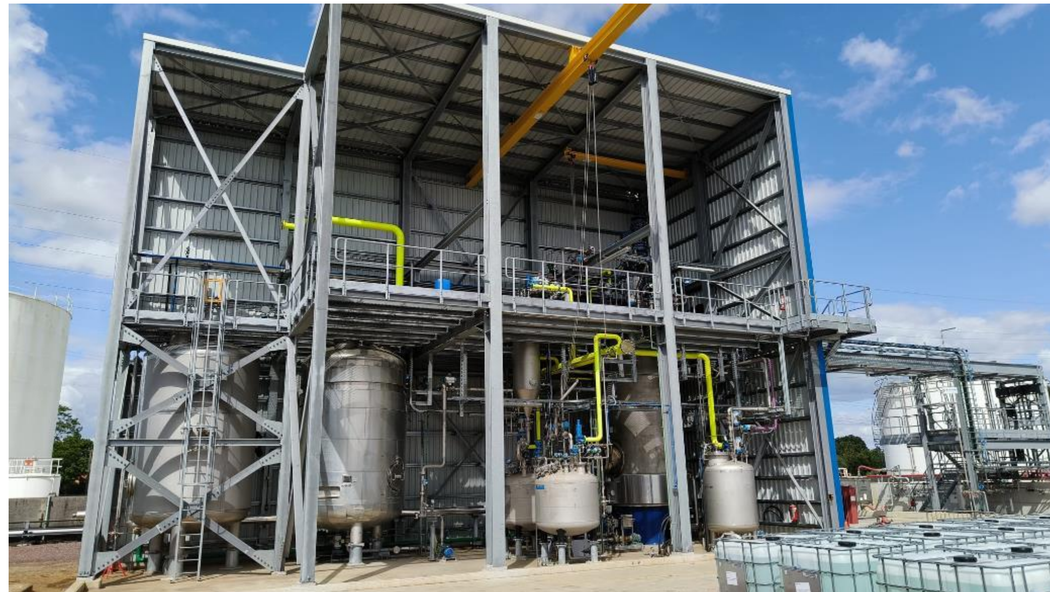
Commercial plant with capacity > 4 kton / year (startup Q1 2025) TRL 4 to 9 during the NewWave project
